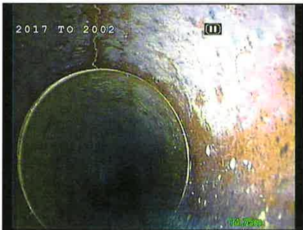
Photo: 5_5a, 00:00:00 14.75m, Crack Longitudinal at 12 o'clock
