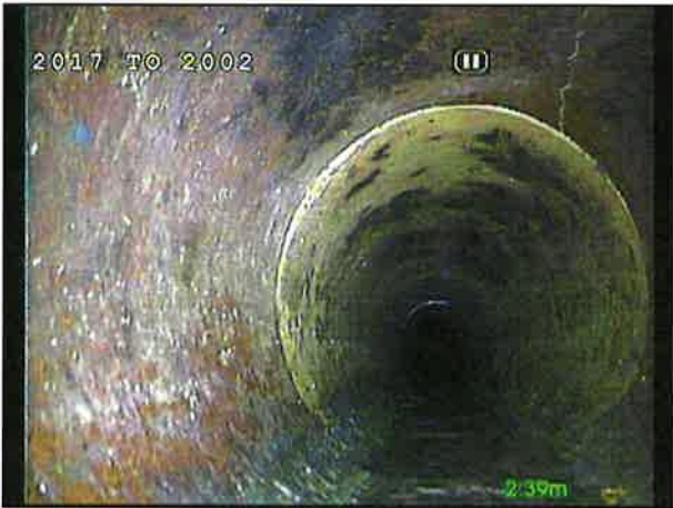
Photo: 2_2a, 00:00:00 2.39m, Crack Longitudinal at 01 o'clock
