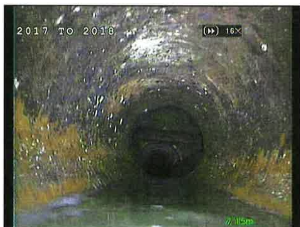
Photo: 10_4a, 00:00:00 6.97m, Crack Circumferential from 03 to 09 o'clock
