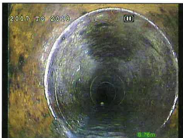
Photo: 8_2a, 00:00:00 0.78m, Crack Circumferential from 06 to 09 o'clock
