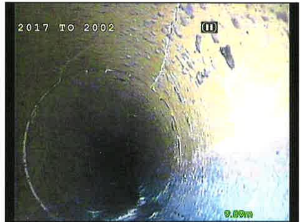
Photo: 4_4a, 00:00:00 9.89m, Crack Longitudinal at 01 o'clock
