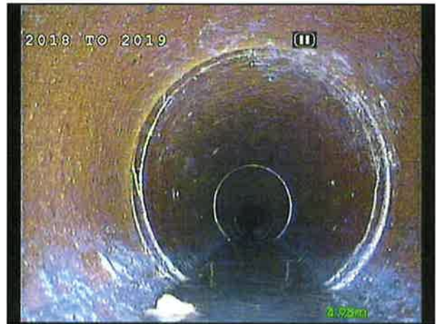
Photo: 18_7a, 00:00:00 4.98m, Crack Circumferential from 12 to 12 o'clock
