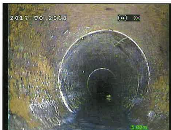
Photo: 9_3a, 00:00:00 5.02m, Crack Circumferential from 01 to 04 o'clock
