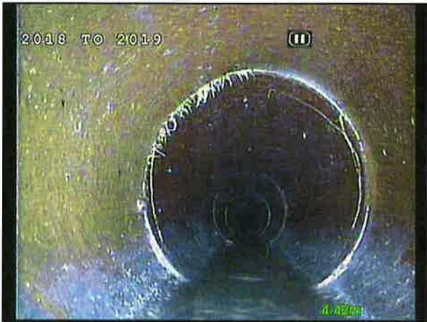
Photo: 17_6a, 00:00:00 4.42m, Crack Circumferential from 08 to 04 o'clock
