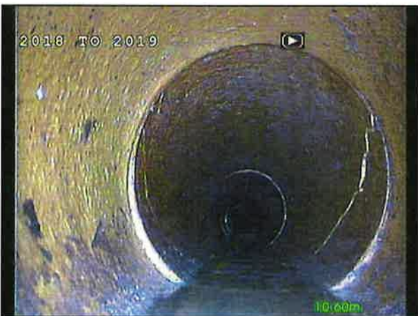
Photo: 19_8a, 00:00:00 10.6m, Crack Circumferential from 02 to 04 o'clock
