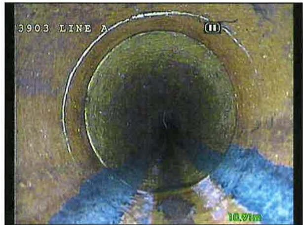
Photo: 13_8a, 00:00:00 10.91m, Crack Circumferential from 07 to 02 o'clock
