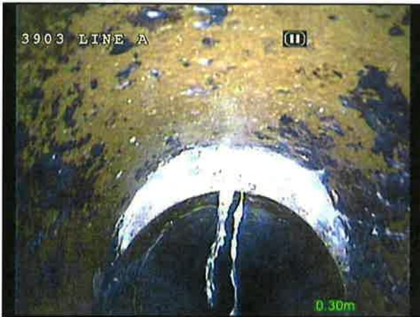
Photo: 7_2a, 00:00:00 0.3m, Joint displaced large, from 09 to 03 o'clock
