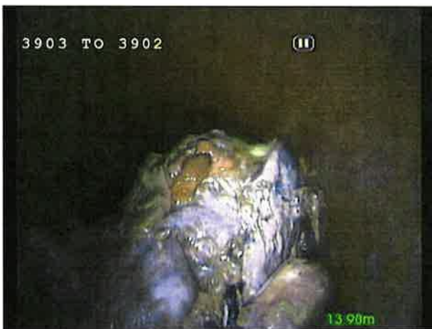
Photo: 4_4a, 00:00:00 13.9m, Other settled deposits 80 % cross-sectional area loss
