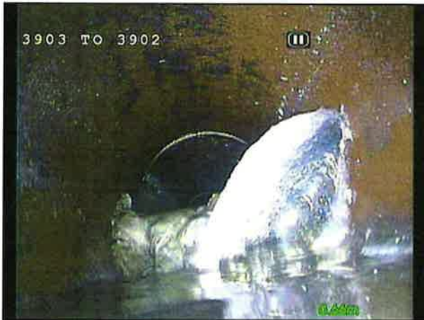
Photo: 2_2a, 00:00:00 0.66m, Other settled deposits 40 % cross-sectional area loss
