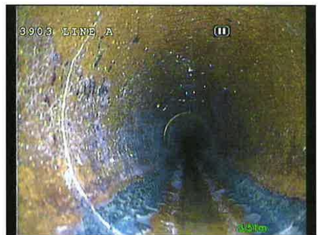
Photo: 11_6a, 00:00:00 3.51m, Crack Circumferential from 06 to 12 o'clock
