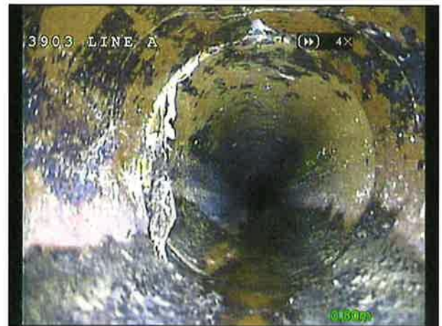
Photo: 9_4a, 00:00:00 0.79m, Crack Circumferential from 09 to 03 o'clock
