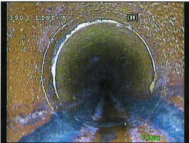
Photo: 12_7a, 00:00:00 7.13m, Crack Circumferential from 07 to 12 o'clock
