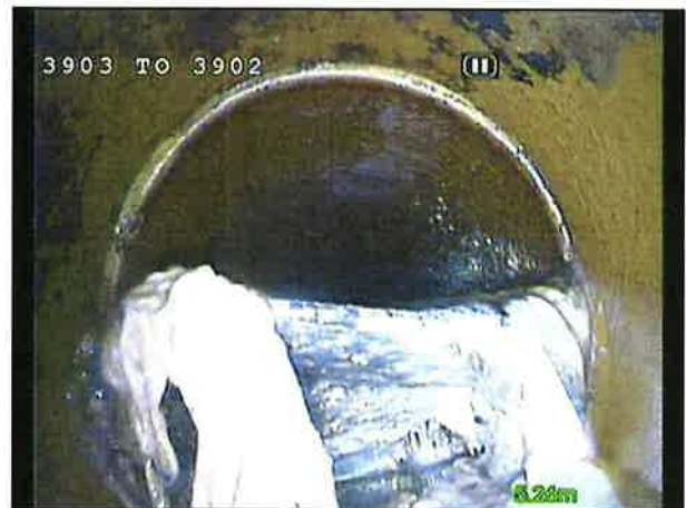
Photo: 3_3a, 00:00:00 5.26m, Other settled deposits 50 % cross-sectional area loss
