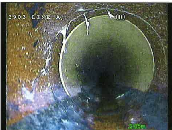
Photo: 10_5a, 00:00:00 2.05m, Crack Circumferential from 09 to 03 o'clock
