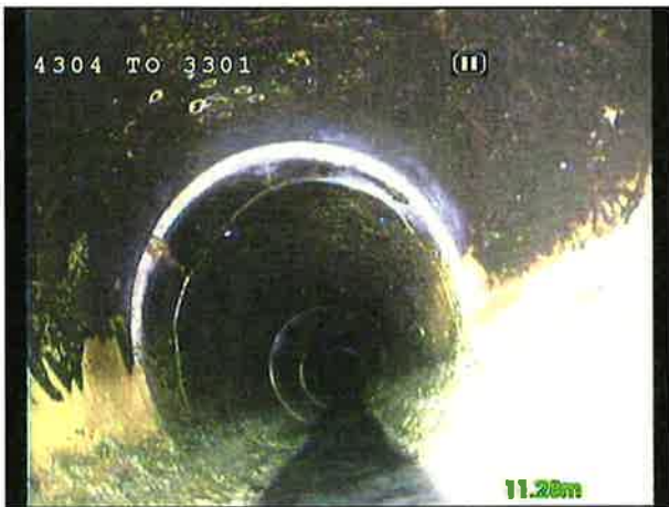
Photo: 4_4a, 00:00:00 11.28m, Crack Circumferential from 07 to 03 o'clock
