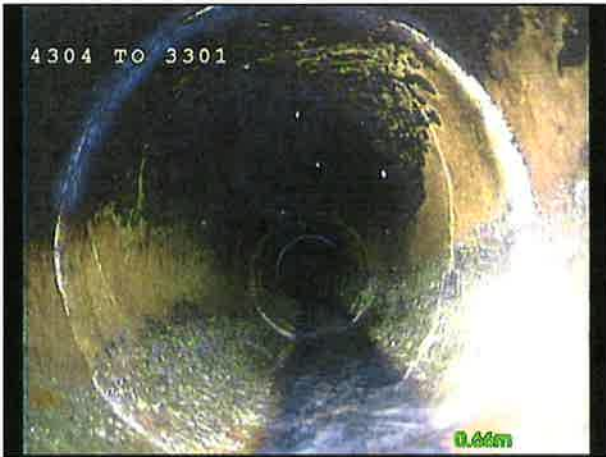
Photo: 2_2a, 00:00:00 0.7m, Crack Circumferential from 01 to 06 o'clock
