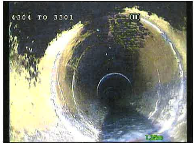
Photo: 3_3a, 00:00:00 1.35m, Crack Circumferential from 02 to 10 o'clock
