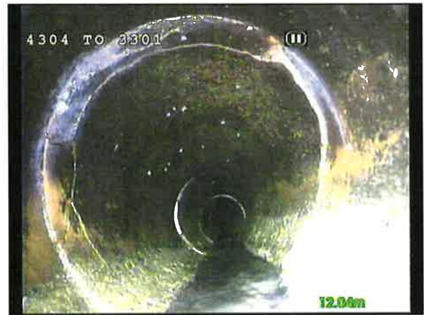
Photo: 5_5a, 00:00:00 12.04m, Crack Circumferential from 07 to 04 o'clock
